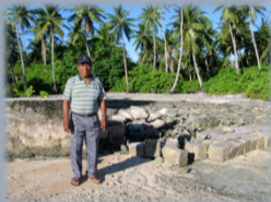
Broken seawall and saltwater inundation, Nanumea
