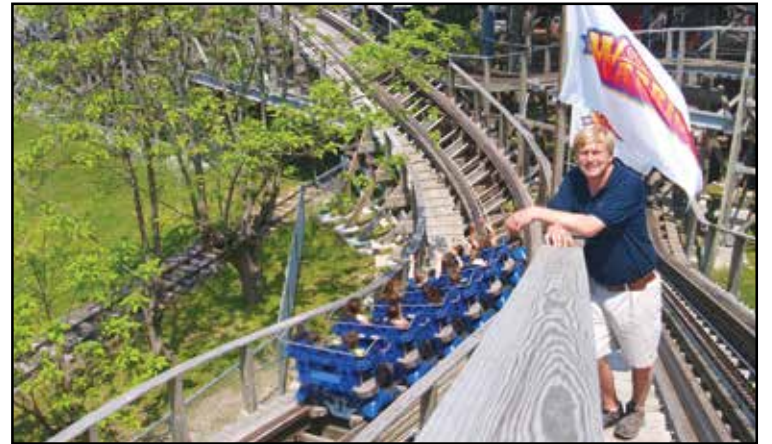
Eric Anderson stands on the lift hill on Wooden Warrior, the marquee ride at Quassy Amusement & Waterpark in Middlebury, Conn. Eric oversaw the building of the much-ballyhooed roller coaster during the 2010-11 construction process. A warrior in his own right, Eric gave up offseason vacationing to see the project completed for an on-time opening. COURTESY QUASSY
