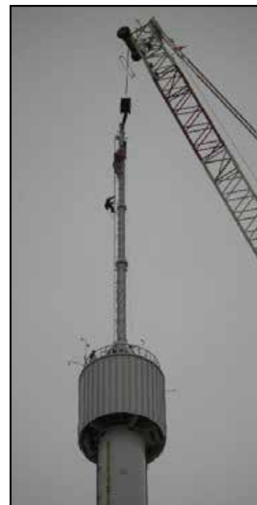
The new 500-foot tall Intamin observation tower for the State Fair of Texas was topped off on Jan. 8. COURTESY ILC
