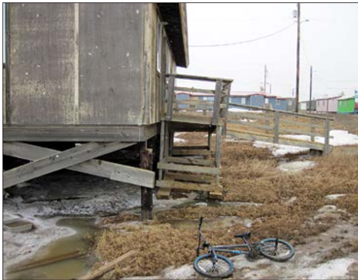
Foundations are impacted by permafrost thaw and heave. Jake Bell, 2014.
