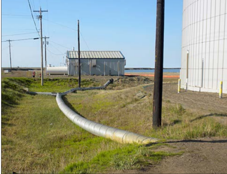
The water line connecting lake and community storage tank. Mike Brubaker, 2013.
