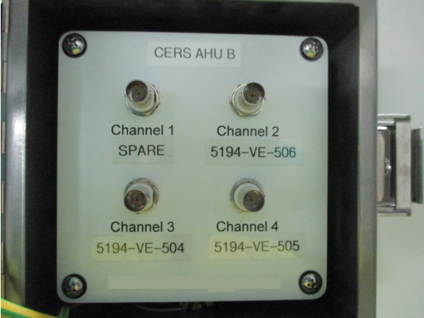
Fig 3. Data Collection Manifold
