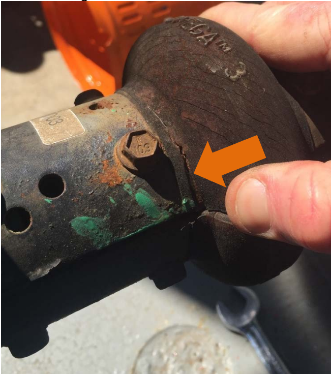
Fig 2. Cooling Pump Coupling Tear
