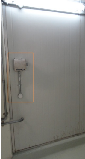
Fig 4. Manifold On Ventilation Fan Wall Panel
