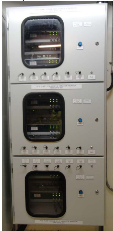
Fig 7. - Bank of Cooling Water Pump Transmitters
