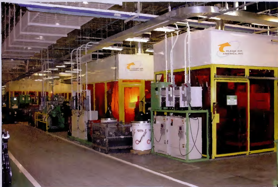
Example of modular air filtration system at F&P Georgia, an automotive parts supplier.
