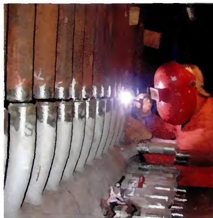
Fig. 3 — Welder Bryan Gray uses the gas tungsten arc process to join the boiler tubes.
