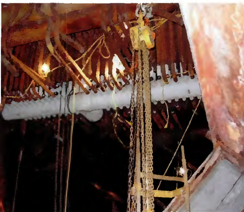
Fig. 2 — The header is shown in place after being hoisted 40 ft to the boiler bay.
