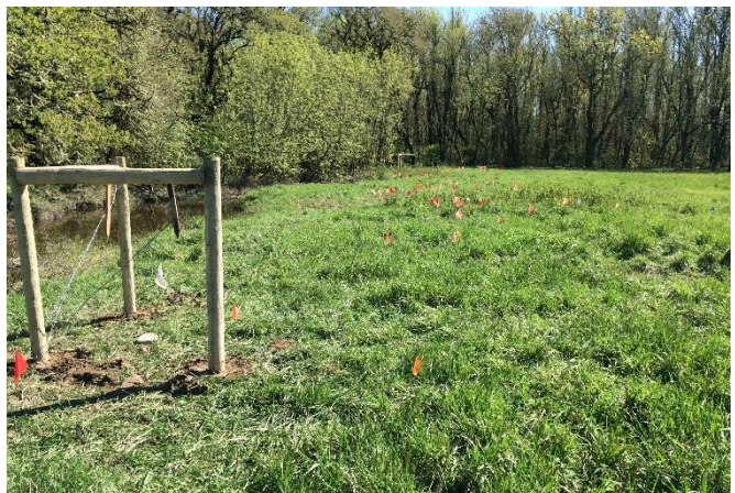
Figure 18. Construction of an enclosure to prevent grazing in Bradshaw's lomatium (flags) habitat at Cutler Lane (May 2016).
