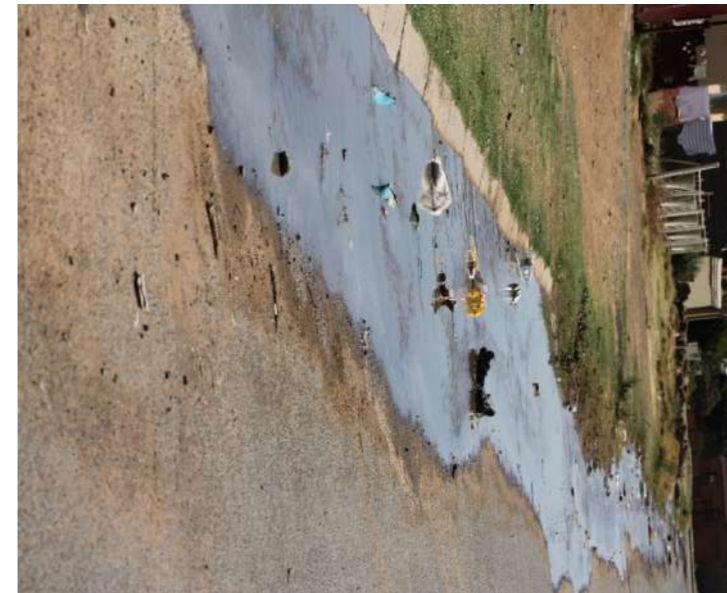
Figure 1: Blocked sewage system and leaking pipes.
