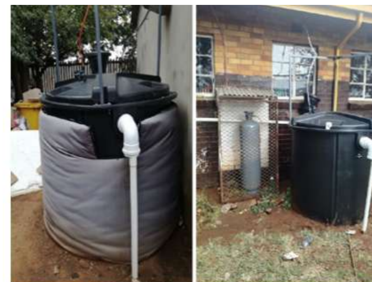
Figure 4: Pre-fab biogas digesters installed at two different schools in Johannesburg (a blanket is sometimes used to maintain a warm temperature inside the digester)
