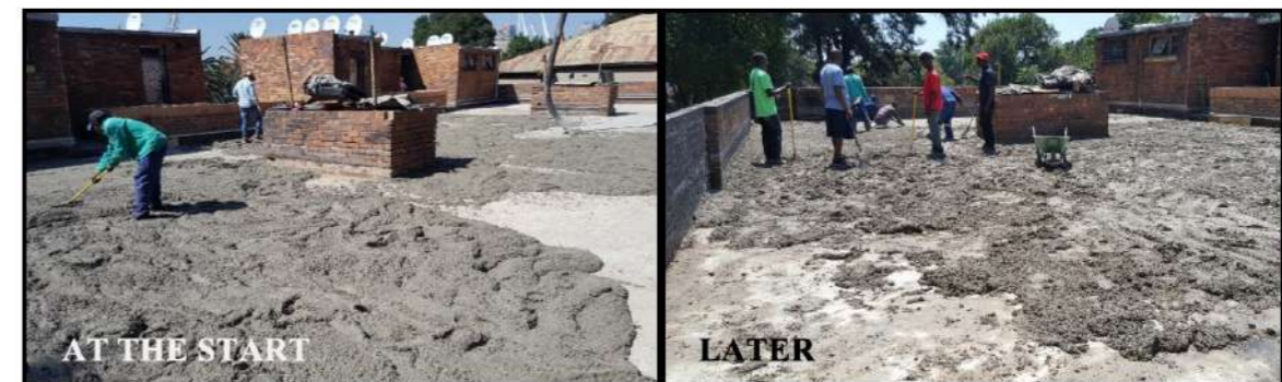
Figure 5: During the process of repairing the screed roof before the waterproofing barrier was installed (Lamprecht, 2019).
