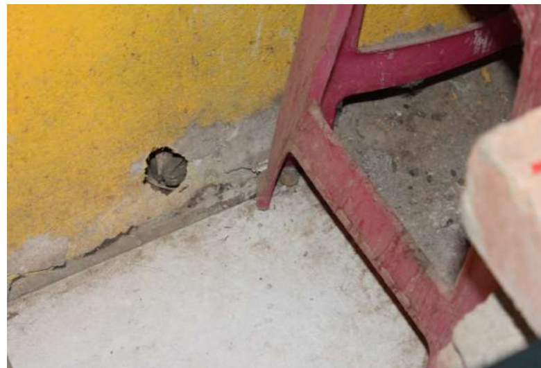
Figure 4: Openings in walls and signs of active rodents (rodent droppings).
