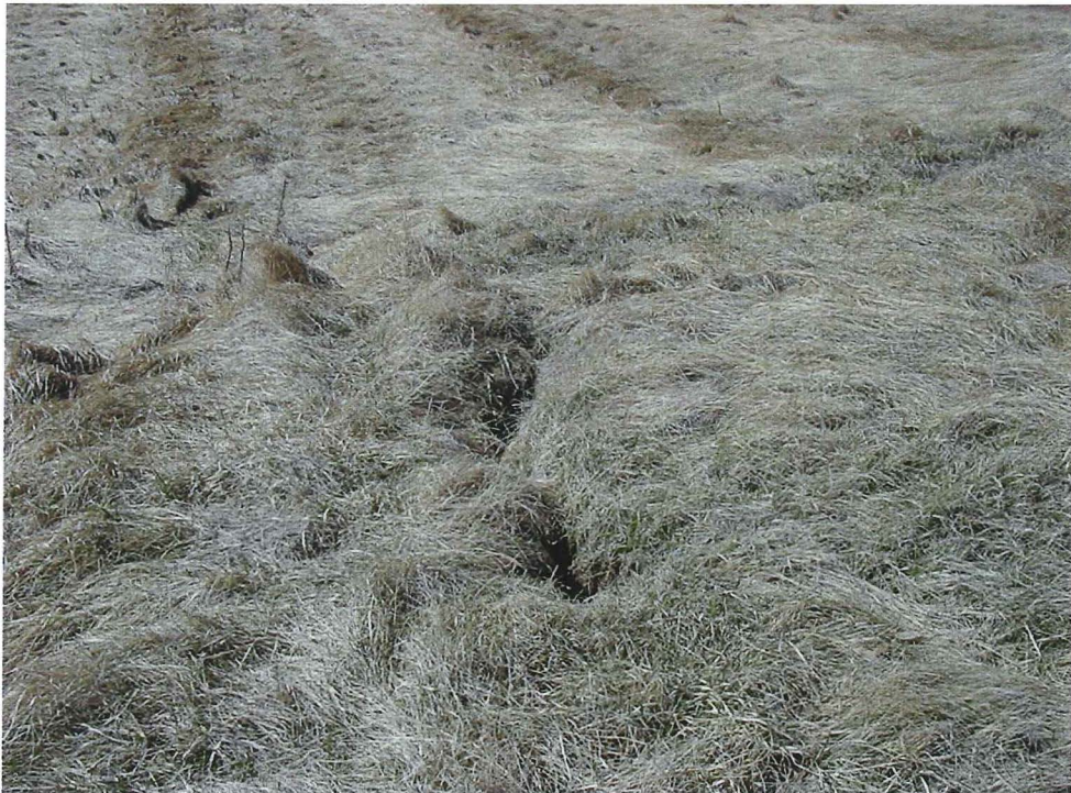
Tear in turf caused by differential settlement East of EW-13 4/3/06
