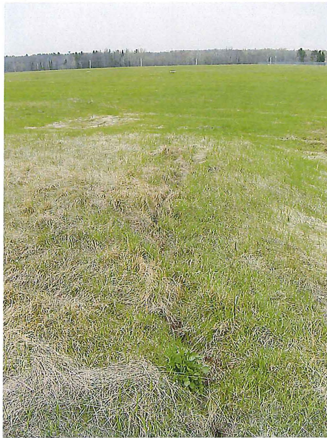
Crack in turf east of EW-13 Looking south-west 05/01/2007
