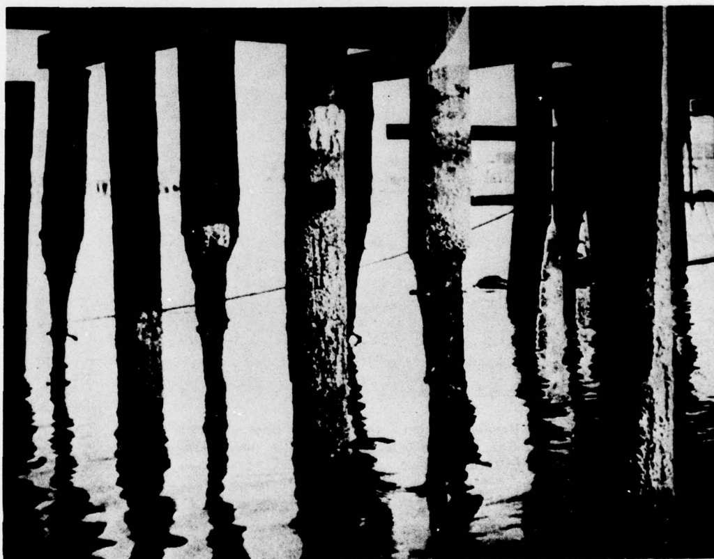
Fig. 2 — Limnorian-damaged piling showing the characteristic damage pattern produced by these organisms in the intertidal zone [1]. Photo courtesy of the American Wood-Preservers Assn.
