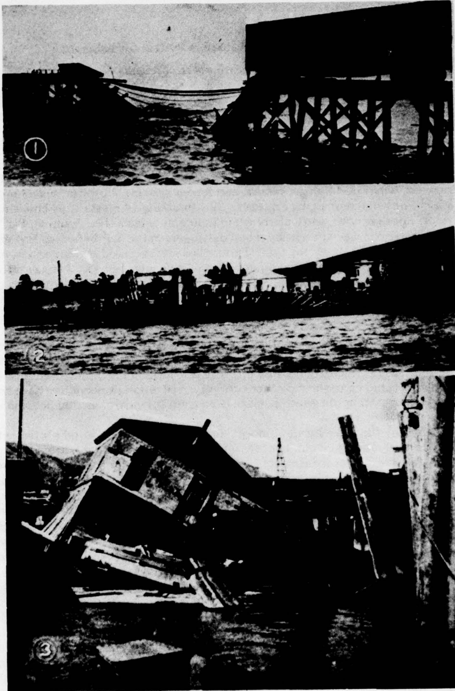
Fig. 1 — Wooden structures in San Francisco Bay destroyed by marine boring organisms: (a) railroad trestle, (b) ferry slip, and (c) municipal wharf and pier [1]. Photo courtesy of the American Wood-Preservers Assn.
