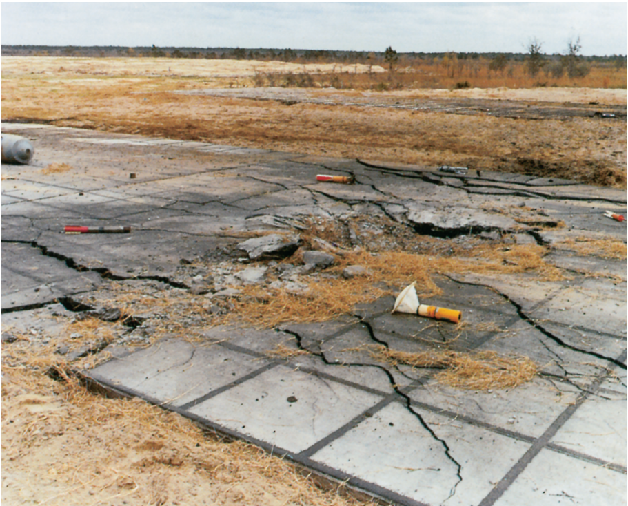
Typical damage to runway for study of landing gear behaviour under operational conditions.
