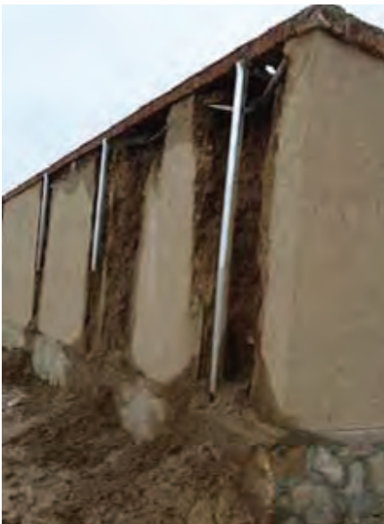
Building deterioration due to water penetration at a Special Police Training Center, February 2013. (National Police Training Center Mentor photo)
