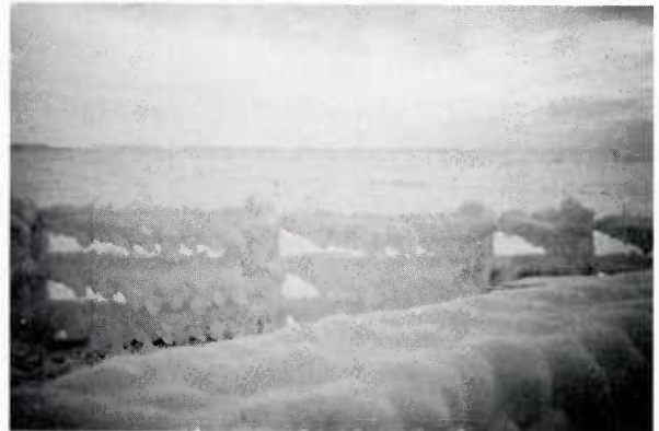
Figure 2-1 Guard rail ice accumulation.
