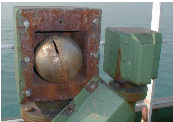
Figure 7 – Air vent head with broken ball float
