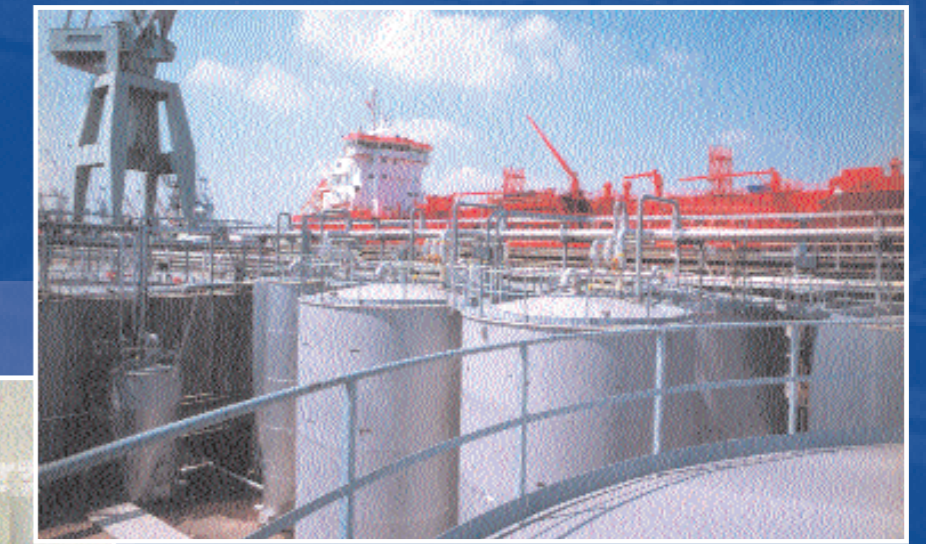
Waste oil storage tanks
