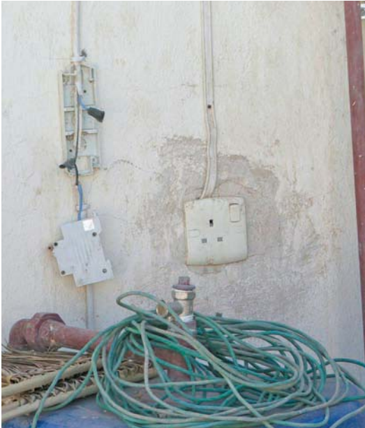
Unsafe electrical wiring and breaker.
