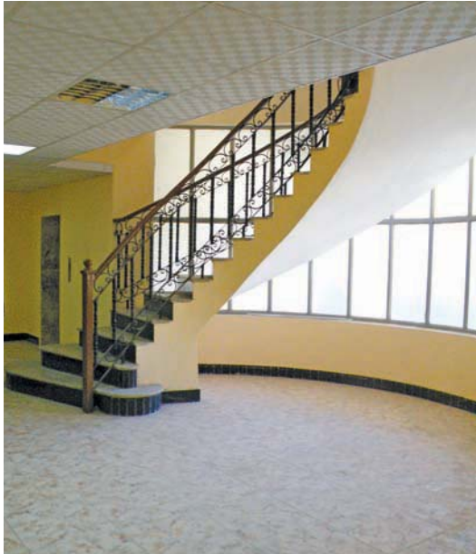
Spiral staircase and SIGIR inspector ducking to avoid the false ceiling.
