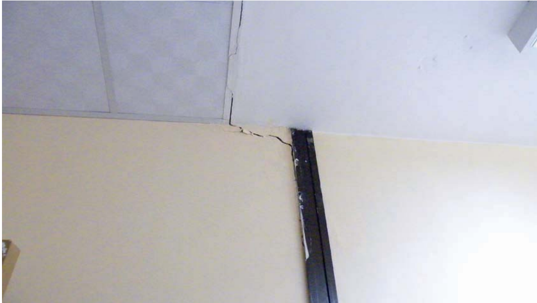
Interior expansion cracks in the witness protection facility.
