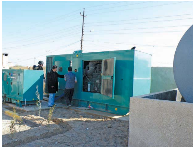
Two generators providing primary and emergency backup power for the Hai Tiseen PHC.
