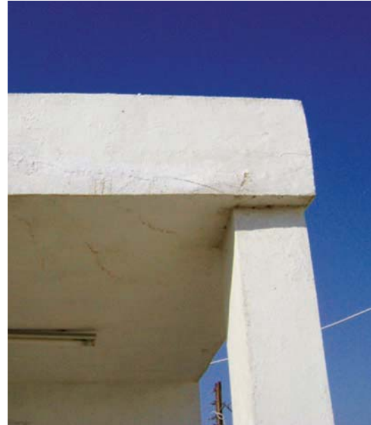
Contractor's "fix" for the reinforcement beam crack: stuff the crack with gypsum and paint over it. (GRC photo)
