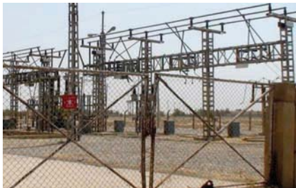
Kirkuk substation. (OPA Photo)
