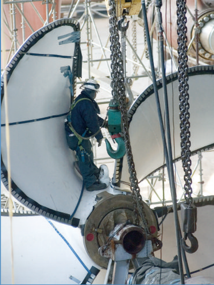
New CVN class propeller being installed on CVN-77. Photo courtesy of Scott Black, NSWCCD Carderock Division.
