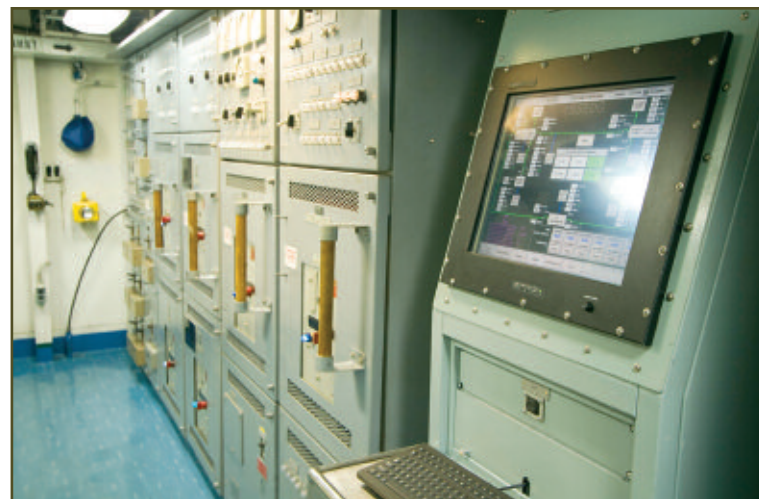
Below: Each diesel generator has one PMP mounted next to its respective switchboard. Pictured is the #1 EDG PMP.
