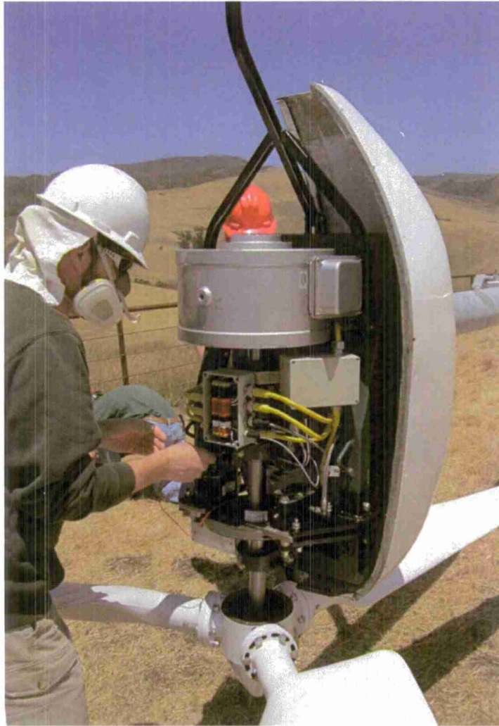
Figure 6: The wind turbine nacelle, on the lowered tower, being serviced by the author in the Spring of 2012. The respirator was used to alleviate allergies.
