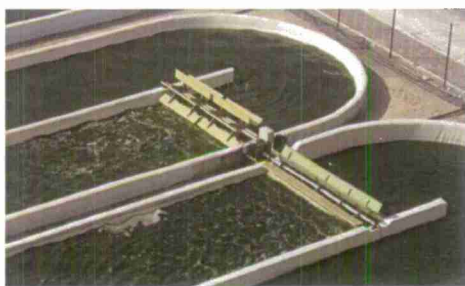
Figure 4: Typical open pond
