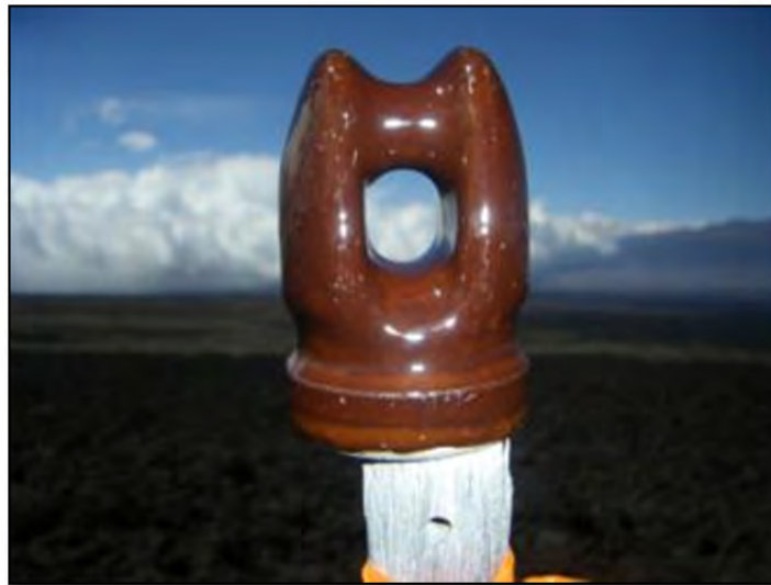
Figure 13. Example of ceramic insulator found on top of communication line poles – West view.
