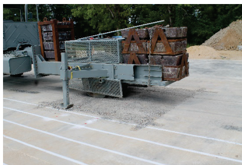
(a) Repair 1-A after 13 passes.
