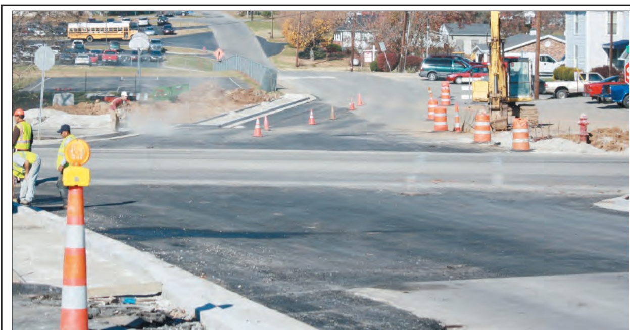
Work on the Newcomb Street - School Street project is beginning its final stages, with the rough coat of blacktop having been recently layed, and the final coat along with the striping set for next week. According to Mayor Gary Cromer, the state still has to put in two of the poles for the lights, and the hospital will soon begin erecting a new sign at the corner of Richmond Street and Newcomb Street.
