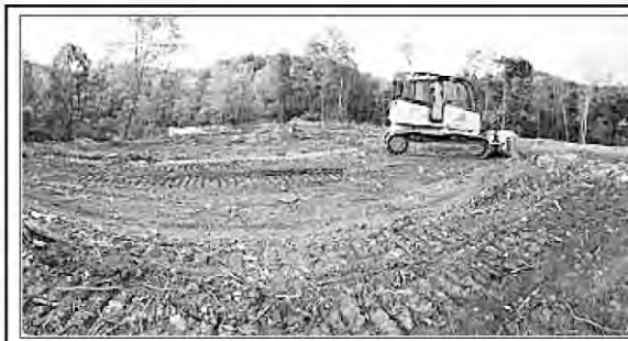
In negotiations with Family Dollar Store for Livingston. Getting the ground ready for construction.
