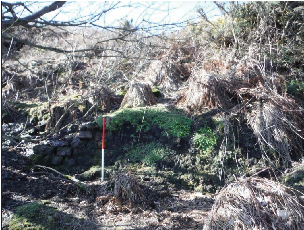
Figure 77- Retaining wall at the base of the working face in the lower quarry floor, looking west (Scale- 1 x 1m).
