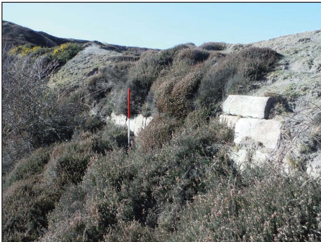
Figure 74- Sandstone retaining wall on the south side of the northern 'arm' of the lower quarry, looking north-west (Scale- 1 x 1m).
