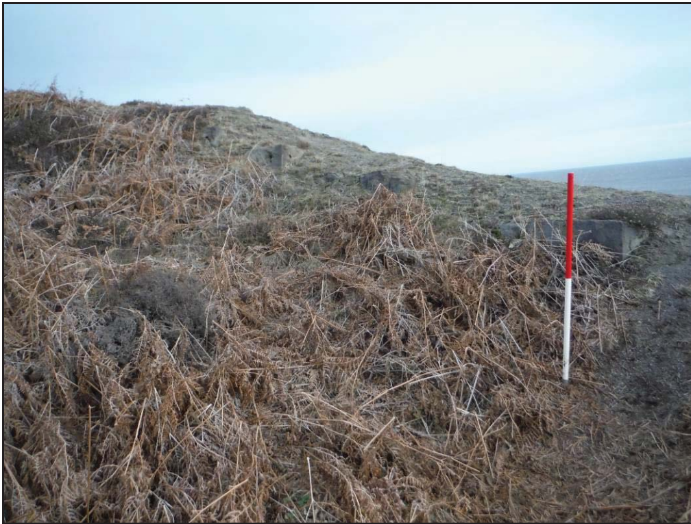
Figure 47- Remains of a stone retaining wall on the western face of the northern 'arm' of the lower quarry area, looking north-east (Scale- 1 x 1m).
