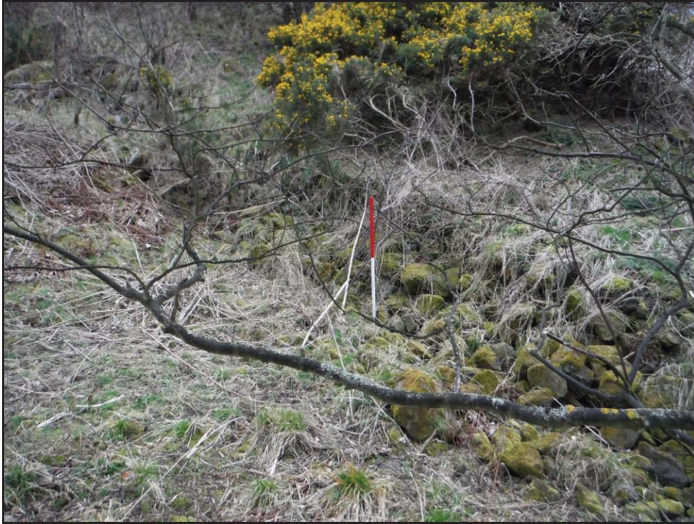
Figure 44- Retaining wall adjacent to a rubble-filled French drain within the quarry floor at Gaytress Quarry, looking north-west (Scale- 1 x 1m).
