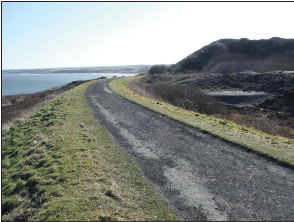
Figure 62- Embanked railway line across the quarry floor of Ness End, looking south-east.
