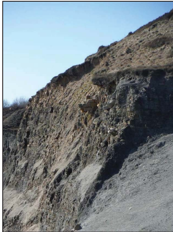
Figure 75- Sandstone wall eroding from the south side of the southern 'arm' of the lower quarry, looking south.
