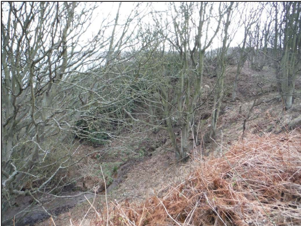
Figure 45- The lower quarry area on the eastern side of the railway line looking south-east. Note water channel entering the quarry floor from a culvert beneath the railway in the background.
