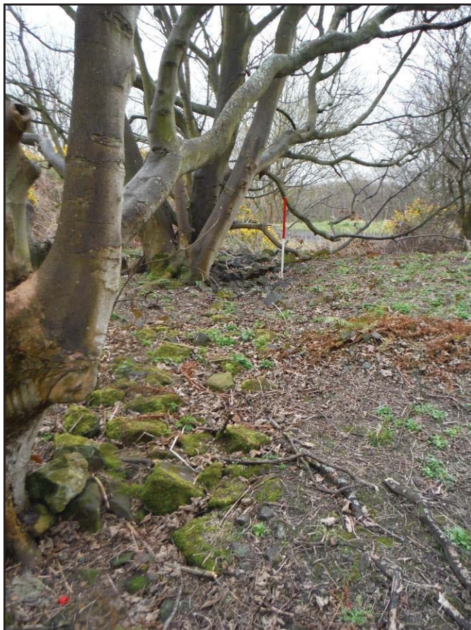
Figure 37- French drain within the quarry floor at Gaytress Quarry, looking south-east. The drain is filled with sandstone rubble in the foreground and slag material in the background.
