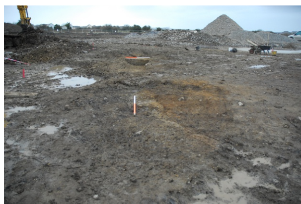
Post-excavation view of posthole F70 in the base of the enclosure ditch to the east, looking west (top)
