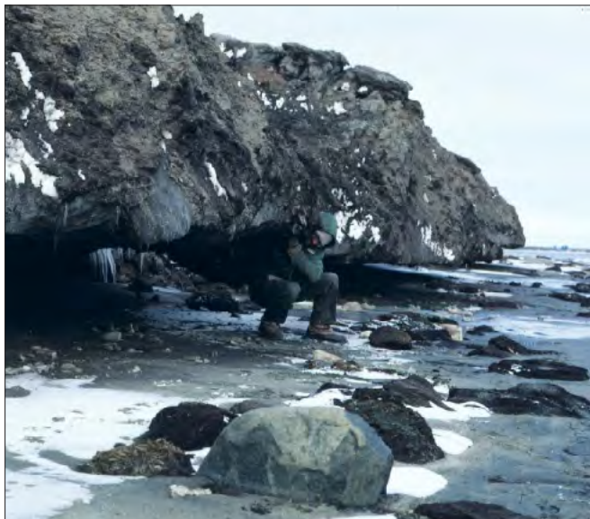
An undercut bluff on the Beaufort Sea coast, the result of a severe storm in August 1980, illustrates the susceptibility of ice-rich coast to rapid erosion. Photo by Catherine Moitoret, Canning River delta, Arctic National Wildlife Refuge.
