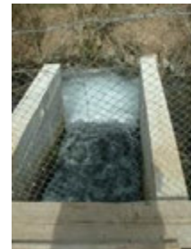
Water outlet, screened for avoiding penetration of otters
