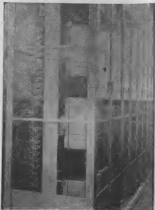
Shown above is one of the three glass cases which contain the heart of the telephone system.
