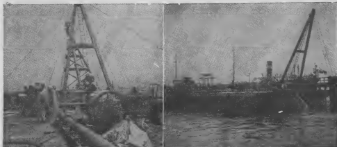
Above at left is a view on the deck of the dredge now cleaning up the Drydock area. At right it is shown in operation.
