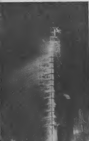
The Welding department puts on a dazzling show during night operations at No. 9 Viscosity Unit stack, as sparks cascade down the scaffolding.
