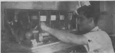
Cornelis Peeren is shown checking the switchboard at the new Watching Service building.
