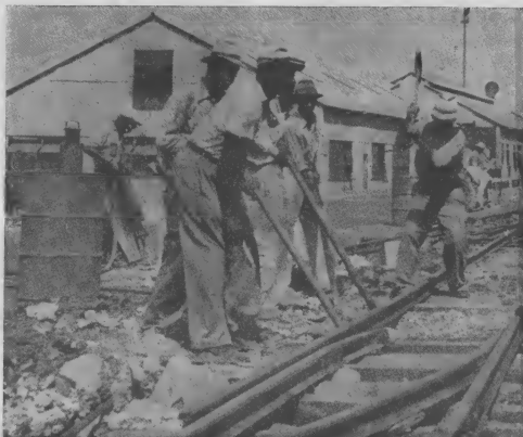
Shown above is the laying of a new section of track between the Dispensary and the M. & C. office, where previously the trains moved along the immediate edge of the auto road. Ten feet of space will now separate them.
