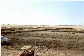
Plate 11. Silage trenches sealed by excavated soil to a depth of 45 cm and finished to provide a camber to ensure run-off from the silo surface
