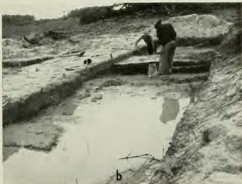
a , Start of work in Fort Walton zone, site J-5; Chattahoochee River in background. b , Trench in Fort Walton zone, site J-5, after rain.
