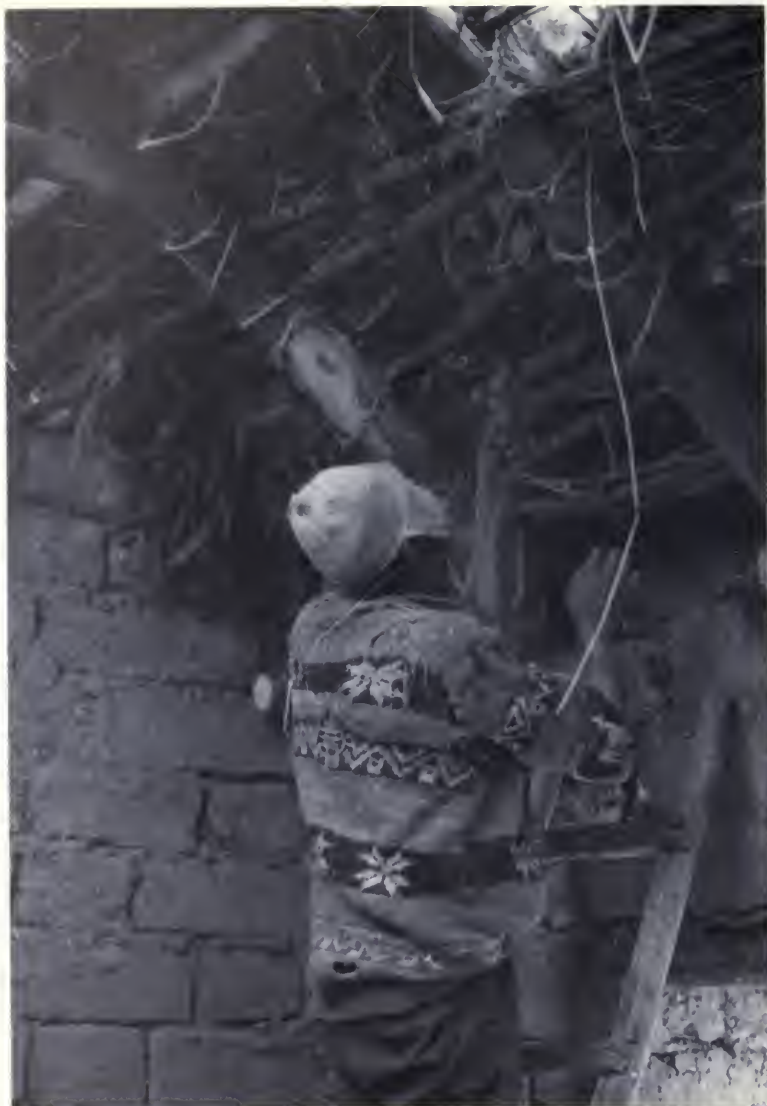
FIG. 30. A.H. thatching a roof. Eucalyptus is laid on the lowermost layer to make the house smell nice. Bundles of ichu grass are sewn onto the purlins with rope made from twisted, pounded grasses (photo CCTC).
