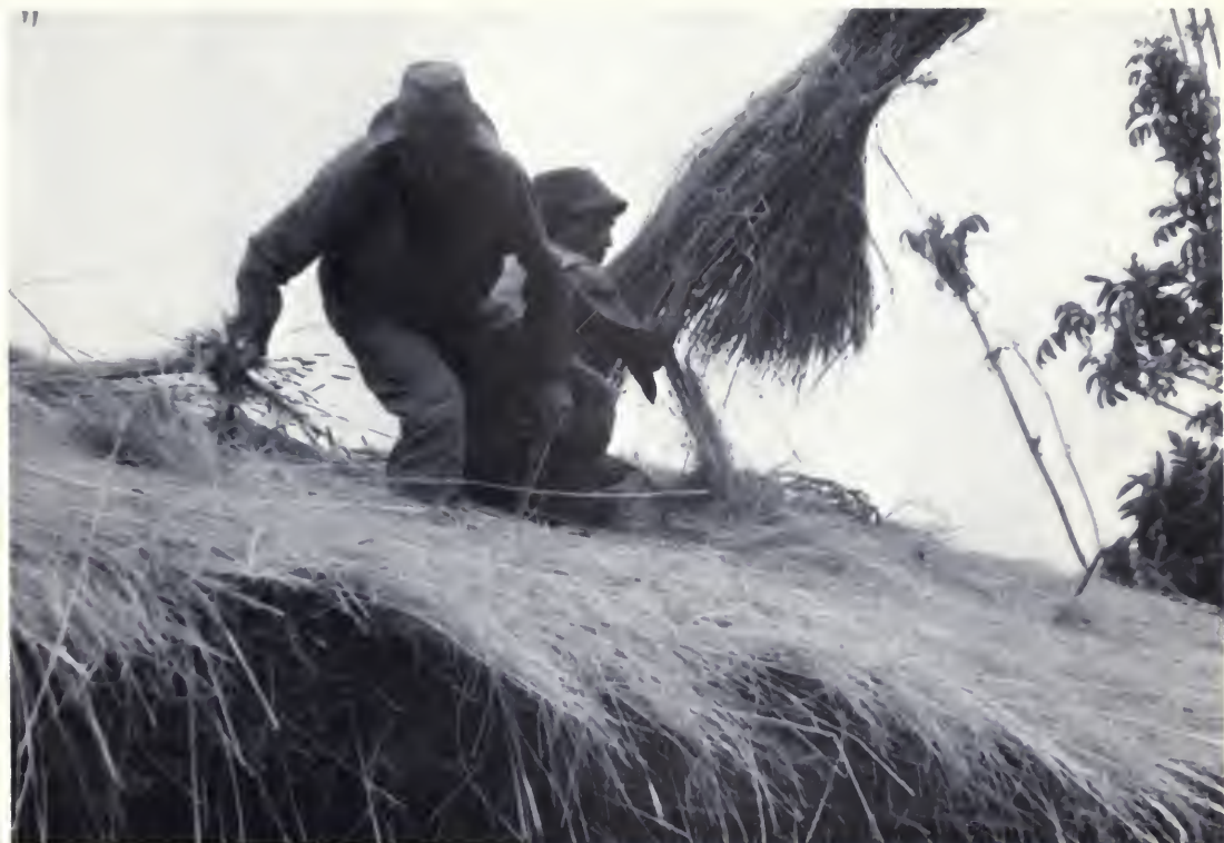
FIG. 29. M.C. and neighbor lay bundles of thatch onto a new roof (photo CCTC).
