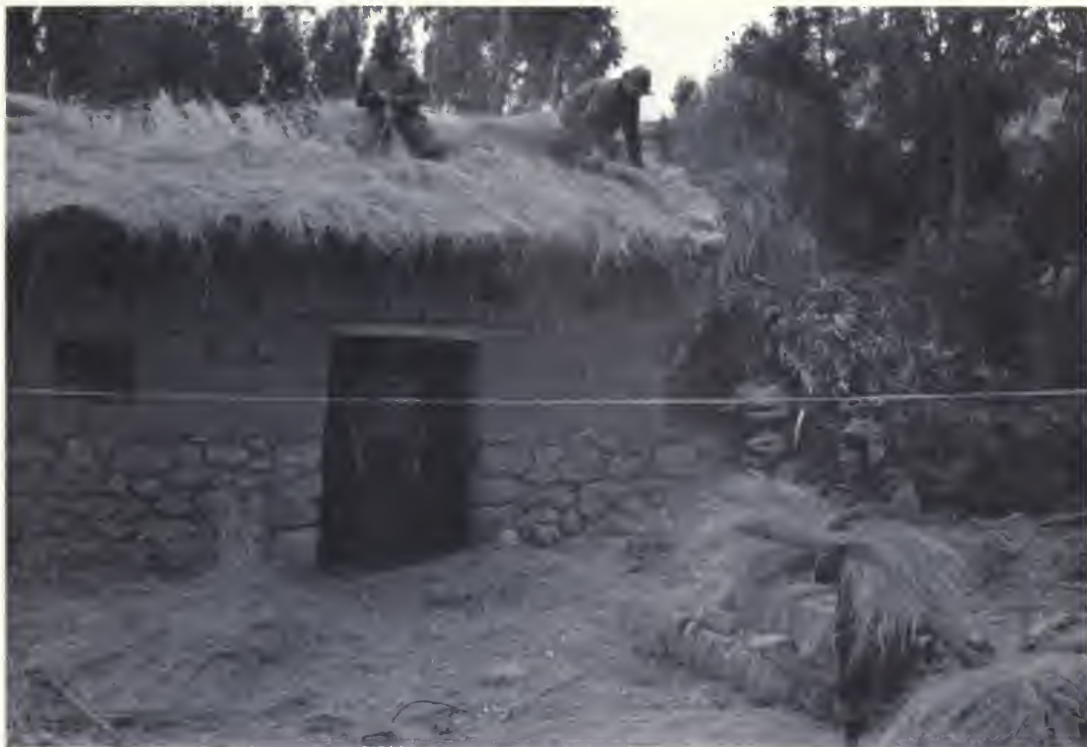
FIG. 8. An ayni group works together to construct a new house (photo CCTC).
