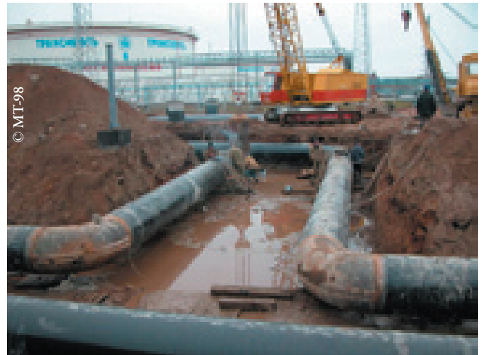
Figure 4.12 Construction of the Baltic Pipeline System with a projected capacity of 62 million tons a year.
