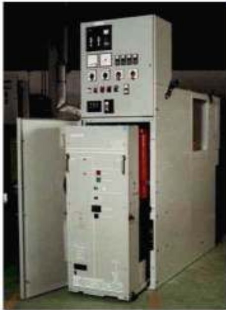
Vacuum circuit breaker (VCB)
