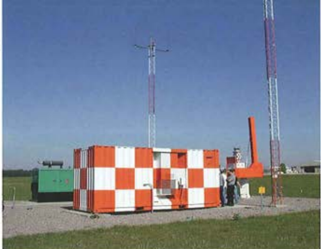
Raytheon has helped with the fixed base precision approach radar or FBPAR facilities such as this one at Fort Bragg, N.C.
