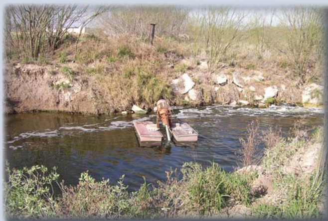
Floating aerator, Mission wastewater outfall
