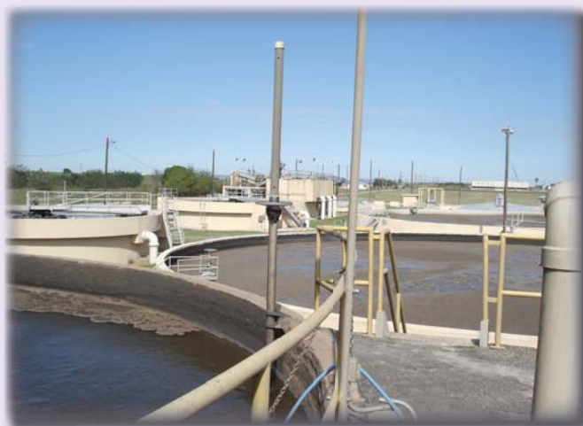
Wastewater Treatment Facility
