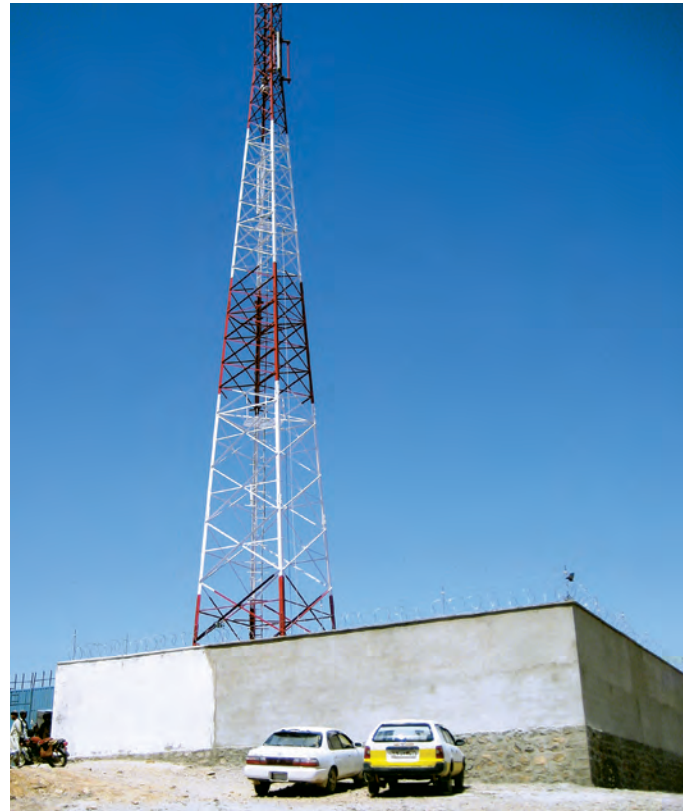
The Roshan cellular telephone tower. Roshan means “light” in Pashtu. The project symbolized the best efforts of the Dutch, U.S. and Afghans to improve communications in the region.
