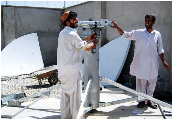
Afghan contractors assemble the cellular telephone tower. Bringing cell phone service to Deh Rawod was a major CA success.
