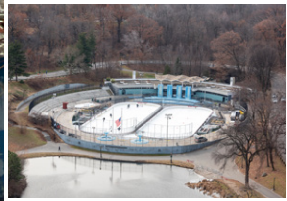
Construction on the Harlem Meer Center began in September 2021; inset: the former Lasker Rink & Pool.
