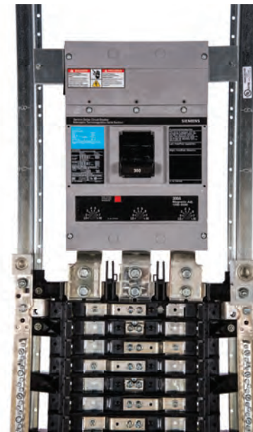
300A Main installed. These Next Gen P1 kits can now be used as top or bottom feed.
