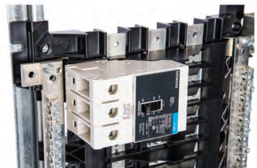
Example of Back-fed NGB Main breaker installed
