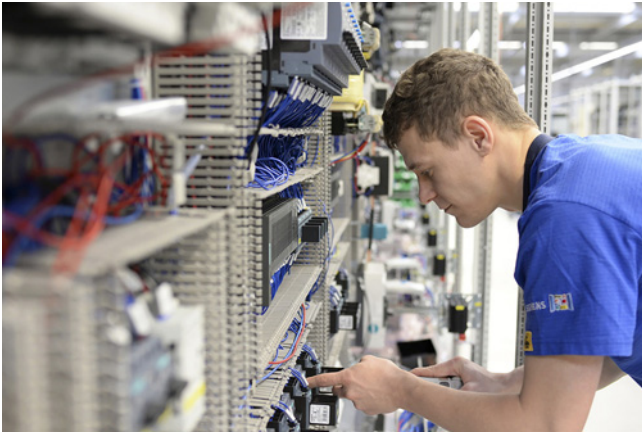
WKC - Control cabinet wiring
