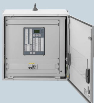
Control cubicle with 7SC80 controller
