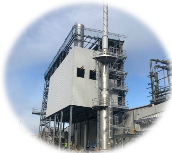
The gasifier plant that could provide the hydrogen-rich Syngas and 98% purity hydrogen.
