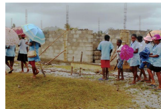
CEG School of the Rural District of Ankofabe in Maroantsetra, Madagascar during rehabilitation after cyclone.
