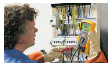
Insulation test at a distribution panel
