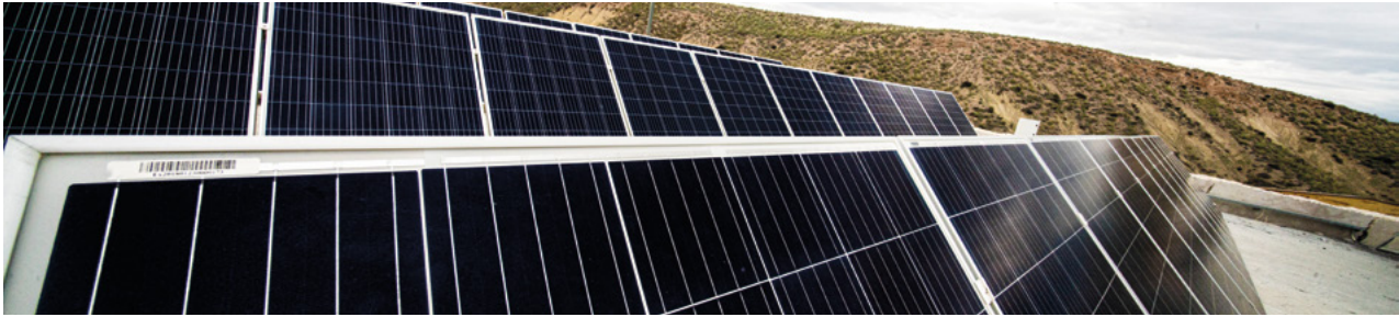
COMA Photovoltaic Solar Plant for self consumption
