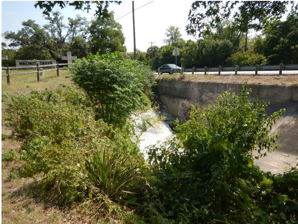
View of a concrete lined unnamed tributary to Walnut Creek facing northeast on July 24, 2018 near the entrance to Walnut Creek Baptist Church.
