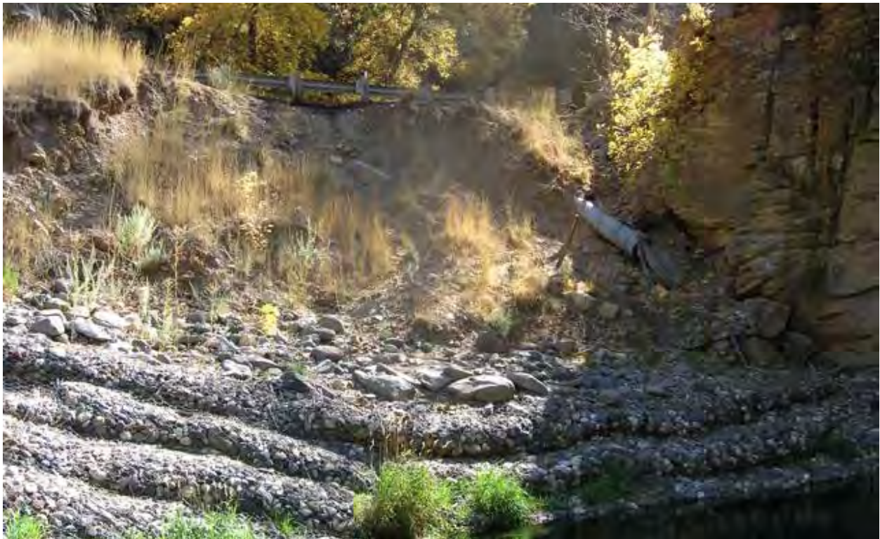
Photo 8. View of the lower end of the project limits (cliff at extreme right), facing south. Note the exposed drainage pipe and the eroded slope to be corrected by the project.
