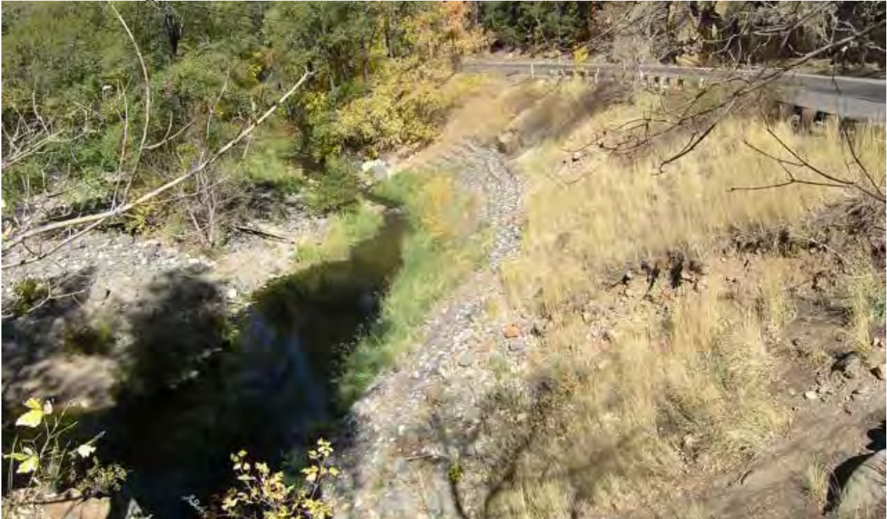
Photo 1. View overlooking the bank protection project site from the driveway of the private property at the top of the cliff at the lower end of the project area, facing northeast. Note the gabion structures on the lower slope and the grass-covered earth slope above.
