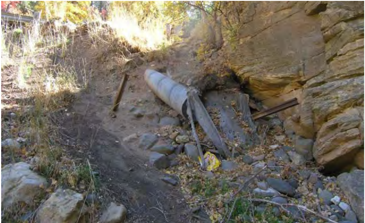
Photo 16. View of the cliff (right), exposed drainage culvert, and eroded slope to be corrected by the project, from the bank of Oak Creek at the lower end of the project area, facing south.
