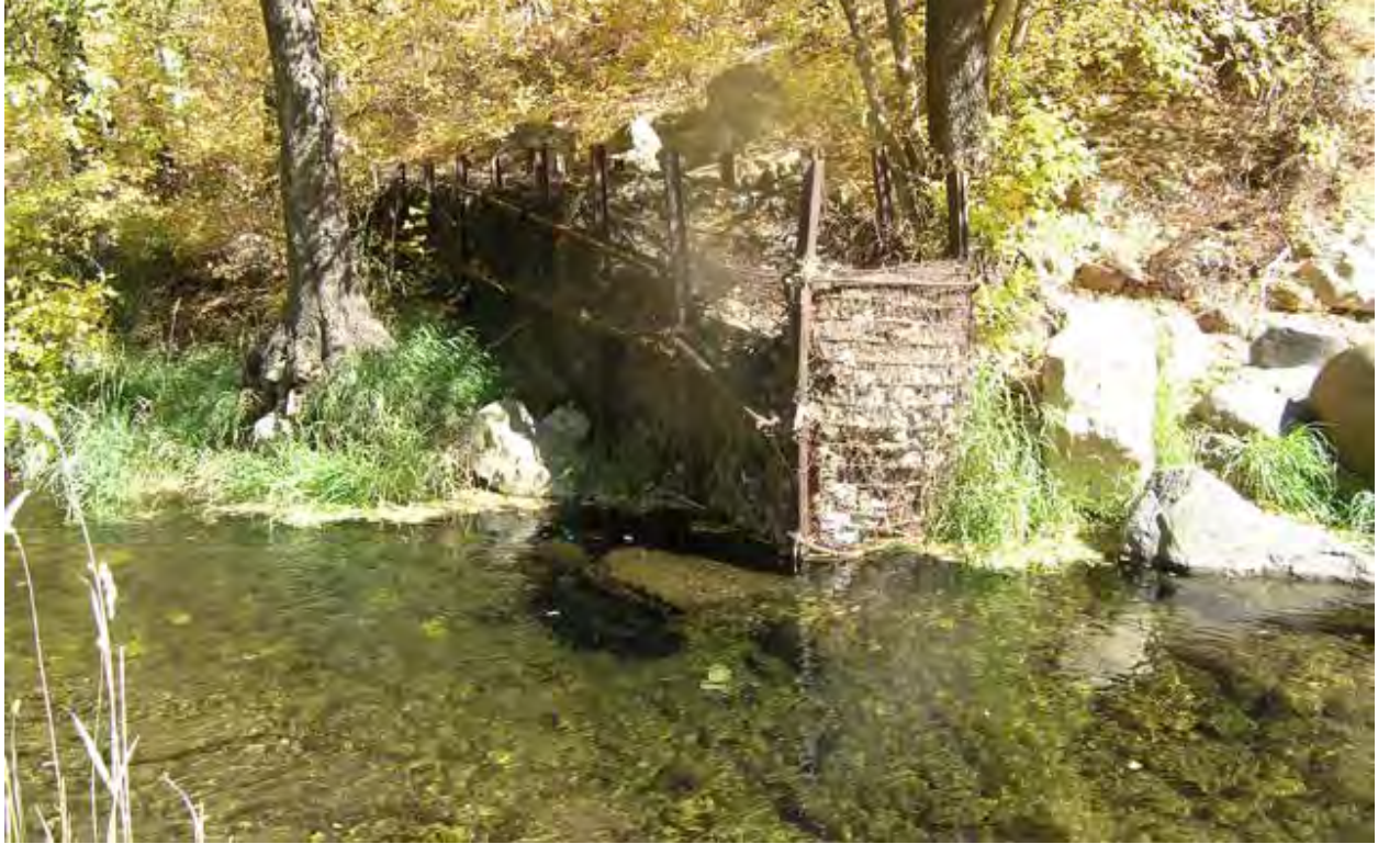
Photo 11. View of the diversion wall from the opposite bank of Oak Creek just upstream of the upper end of the project area, facing east.
