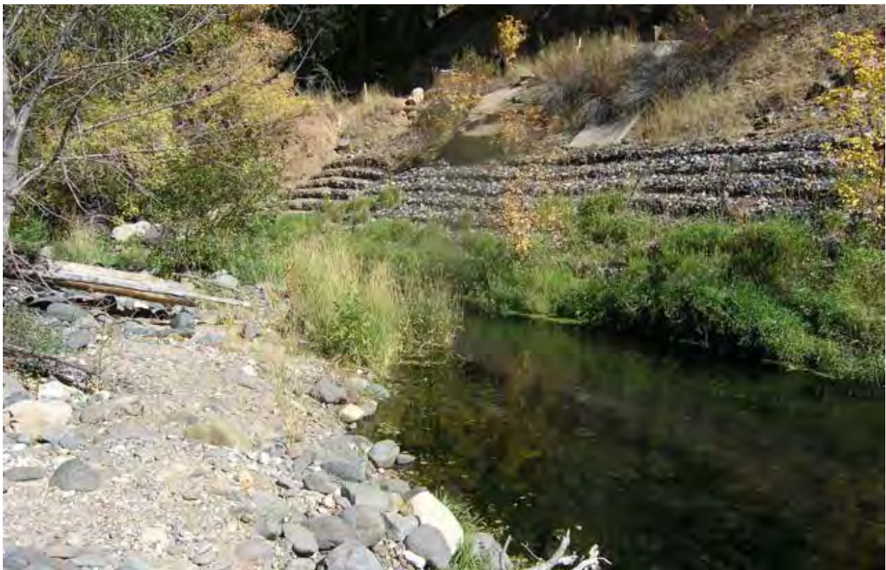
Photo 6. View of the upper end of the project area from the opposite bank of Oak Creek, facing east. Note the cement spillway (to be removed) above the gabion structures (center right).
