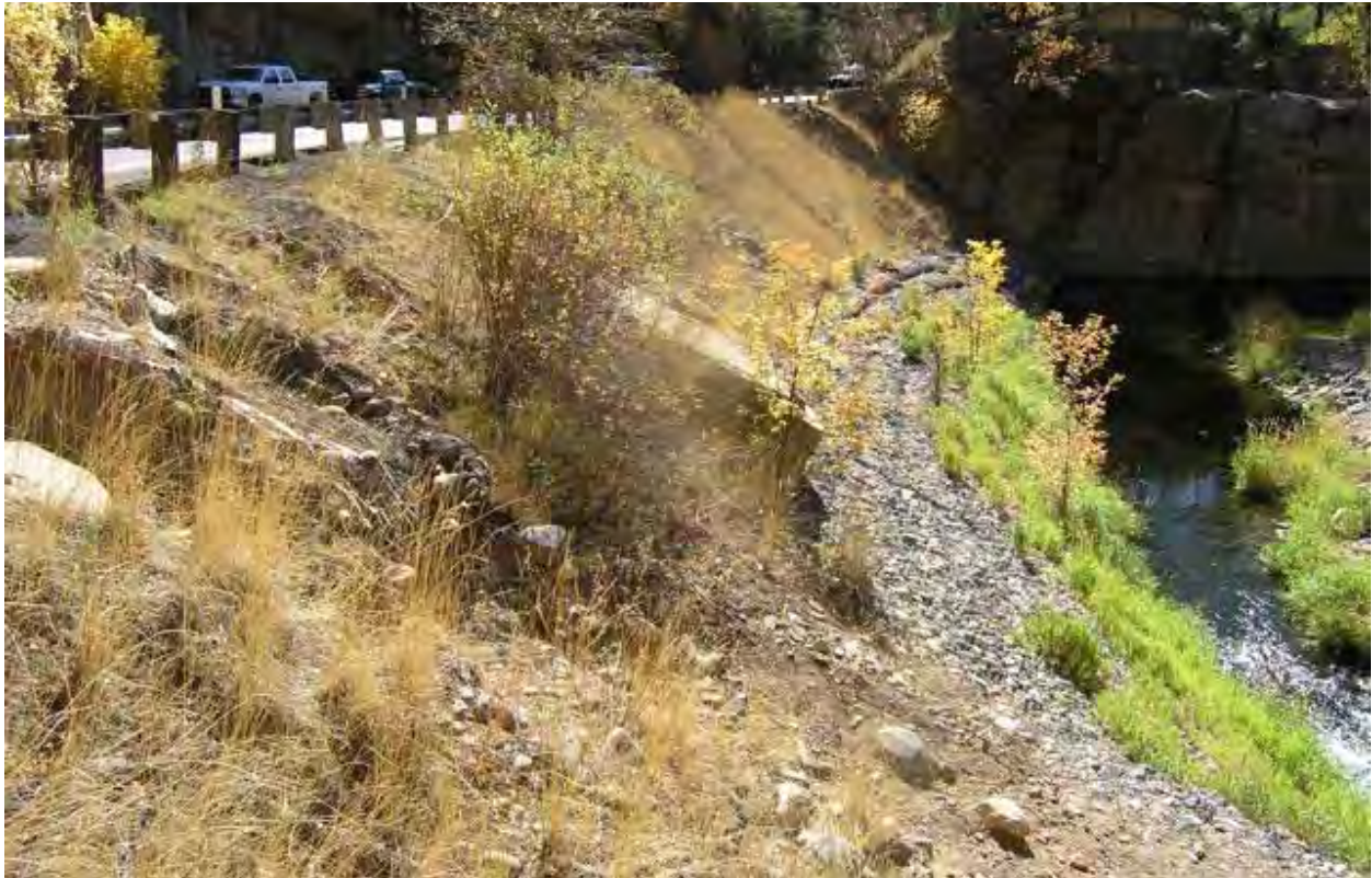
Photo 14. View of the project area from just off SR 89A, facing southwest. Note that the project will extend gabion structures from the existing structures to the roadway. Work will occur on the open, relatively unvegetated slope.
