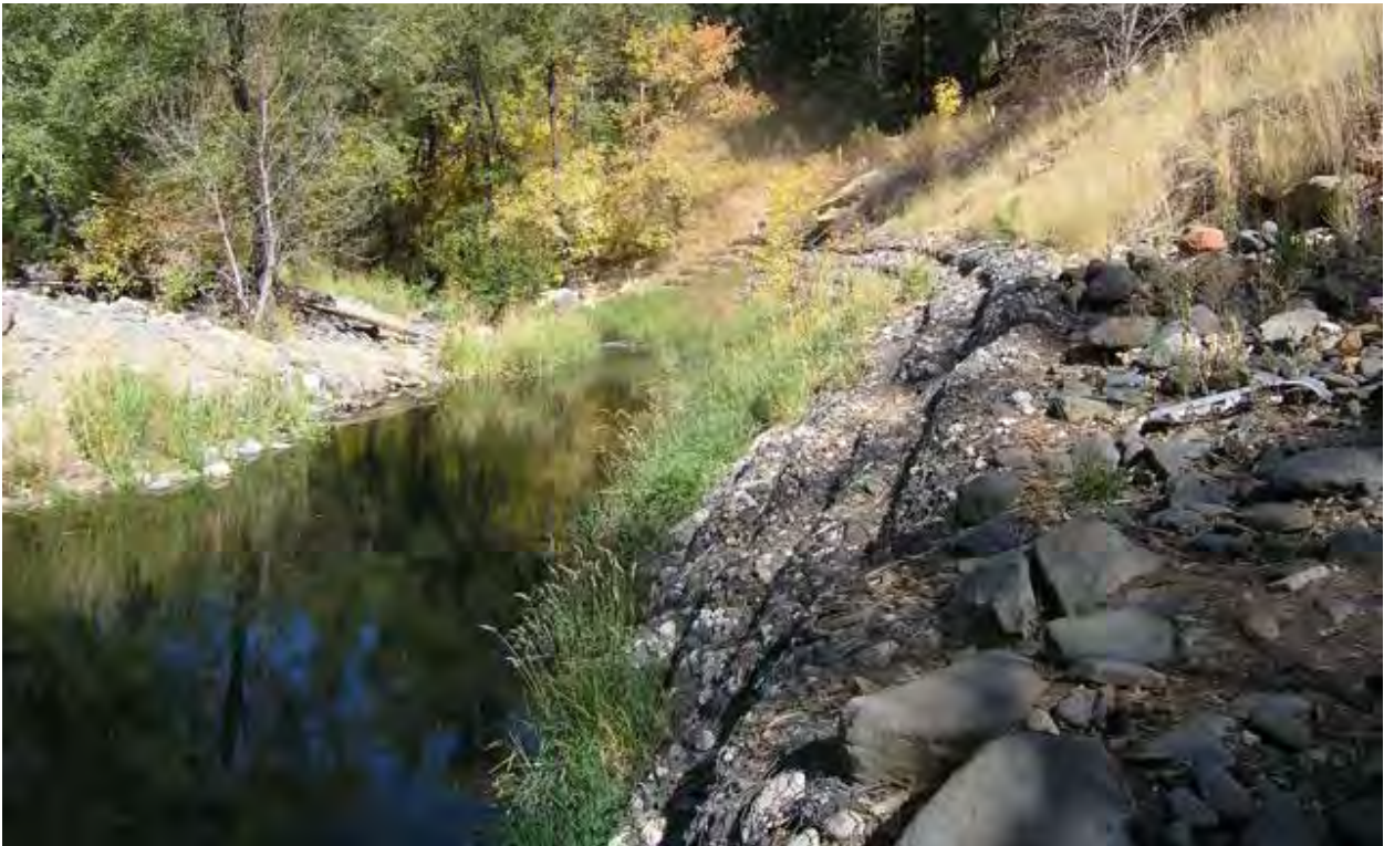
Photo 2. View from the base of the cliff and the lower end of the project area, facing northeast. Note the gabion structures on the lower slope and the grass-covered earth slope above.
