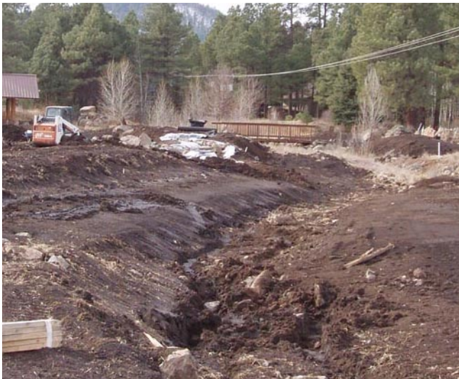
figure 3 Construction of Willow Wash in 2008. The hardscaping phase exposed a large amount of soil, but created the necessary features for the riparian habitats.
