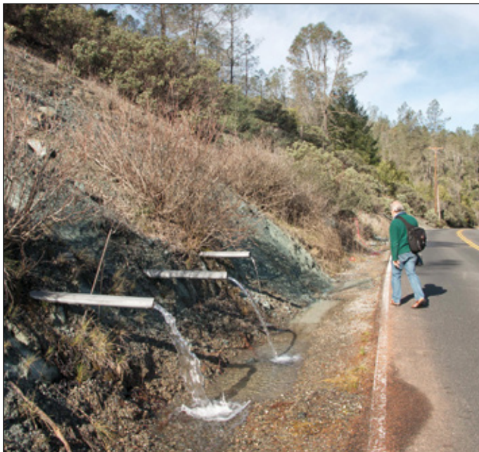
Figure 52. Drainage pipes in serpentinite (Mile 3.8). Serpentine soils retain water very well and these drain pipes can flow even in dry years.
