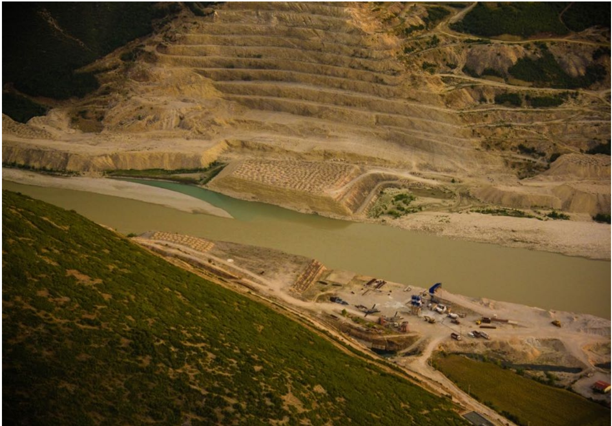
Abandoned construction site of the Kalivac dam on the river Vjosa in Albania. In 2017 a new concession was issued to Turkey's Ayen Enerji & Albania's Fusha to re-start the project. Photo: © Roland Dorozhani
