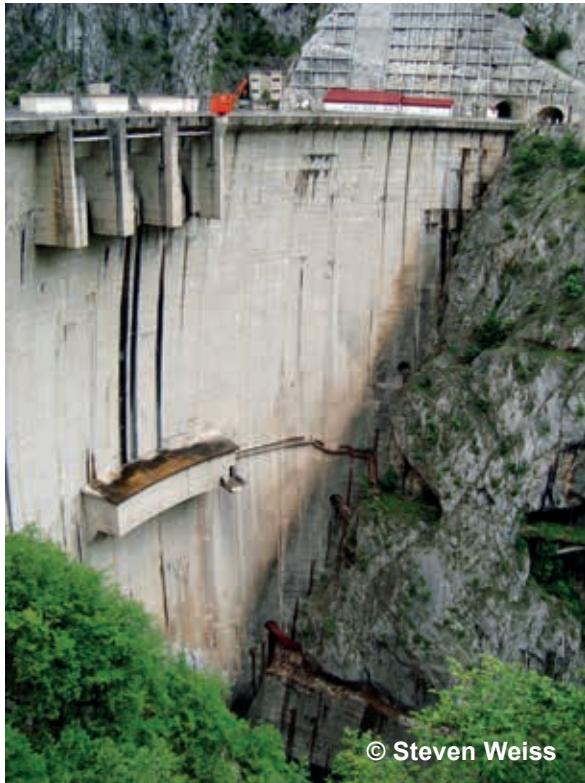
Fig. 2. Left, the 228 meter high Mratinje Dam on the Piva River, Montenegro; Right, the 113.5 meter high Krichim Dam on the Vacha River, Bulgaria.
