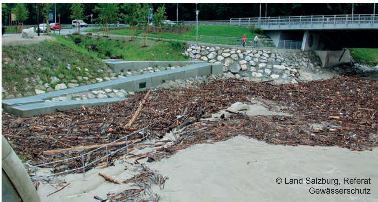
Fig. 10. Debris jam on the downstream side of a vertical fish pass on the Saalach River, Austria. (BMLFUW 2012).
