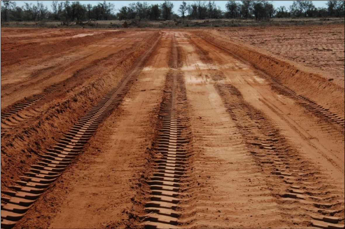
Plate 1-02: Topsoil stripping at the Snapper Mine. At this location the 'white' of the B horizon carbonate layer can be seen emerging in the middle of the laser-scoop cut at the mapped depth and planned cutting depth of 30cm.
