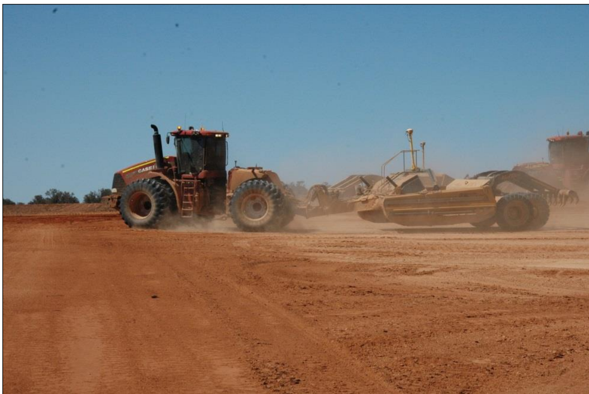
Plate 1-01: A 4wd tractor towing a laser scoop bucket with differential GPS mounted on-board undertaking topsoil stripping at the Ginkgo Mine. These machines have accurate control in soil stripping operations, but care has to be taken to avoid stripping of underlying calcareous subsoil in topsoil stripping operations.
